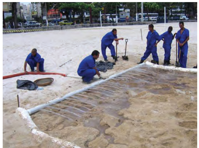
▲ Figure 1: Cleaning of oiled sand in-situ by low pressure flushing, with sorbent boom deployed appropriately to capture released oil.
